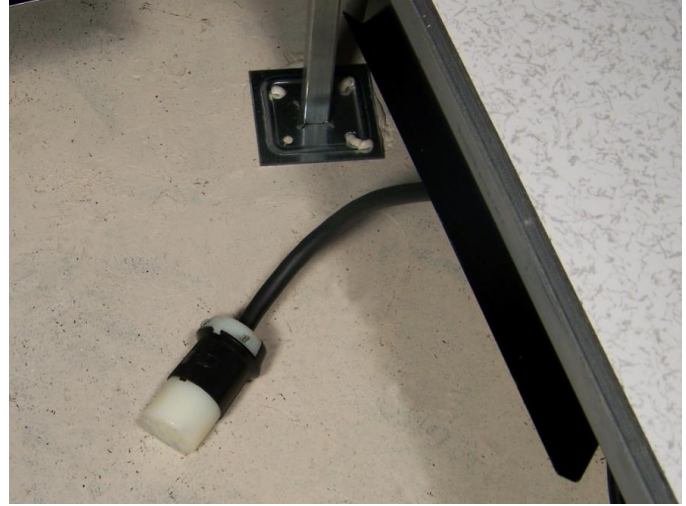
Figure 6 – Power Outlet from Site Source
