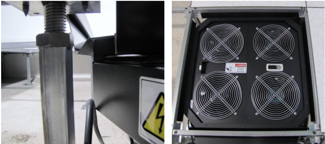
Figures 8,9 - Installation of PowerAire® Quad Unit onto Tool Less Hangers
